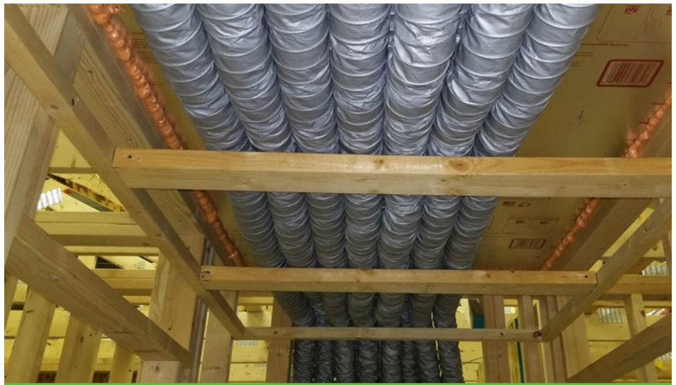
Figure 1. Smaller diameter homerun duct system inside a house.
