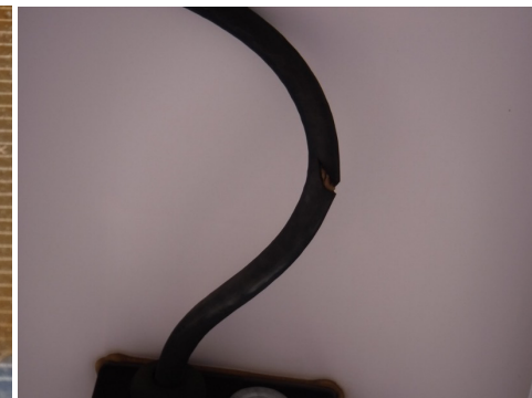
Cracked cable from J-box
