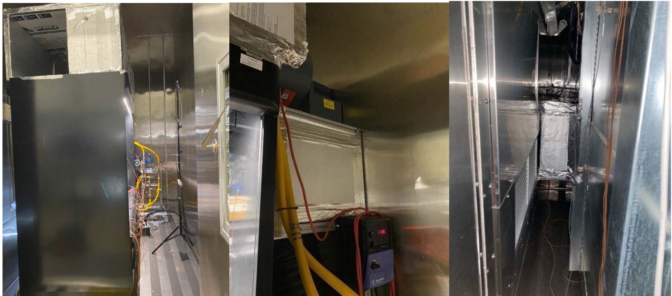
Figure 10. (Left) Baffling System Used to Direct Condenser Rejected Heat, (Center) Booster Fan, (Right) Baffling Discharge to the Chamber Return Grille
