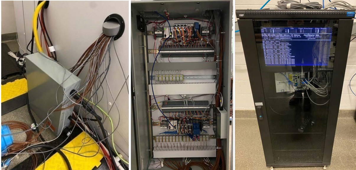
Figure 11. (Left) Wattnode “Meter Box” to Measure Component Power, (Middle) Data Acquisition System Terminal Panel, (Right) Communication Interface for Data Acquisition System
