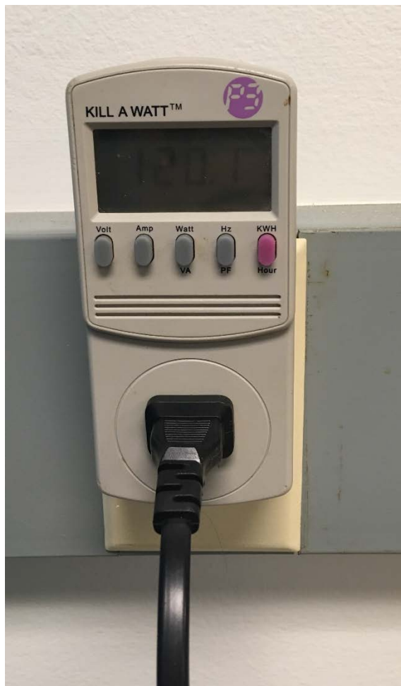
Figure 28. Example of a plug load monitor
