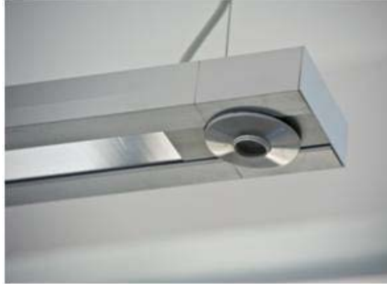
Figure 36. Light sensor for daylighting in NREL’s Research Support Facility
