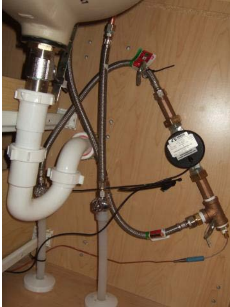
Figure 47. A turbine flow meter, installed under a sink, is used to measure the hot water flow rate and total usage
