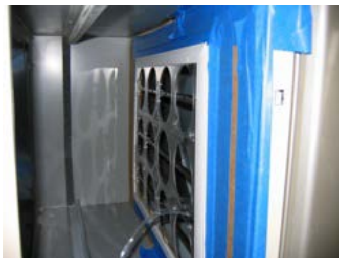
Figure 13. Orifice plate in use
