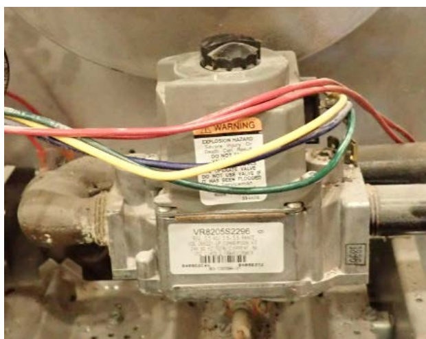
Figure 57. Close-up of the solenoid valve and wiring
