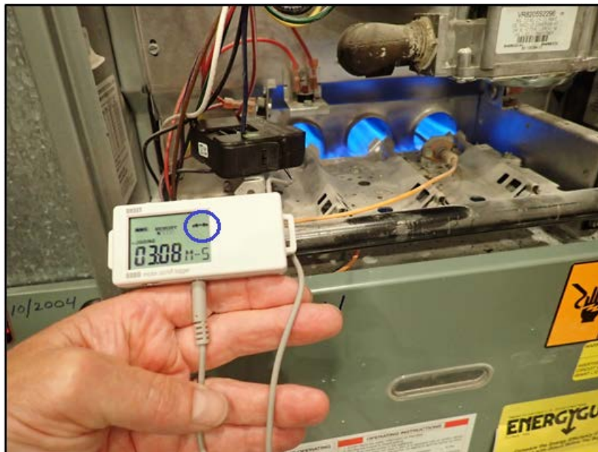
Figure 59. Example installation using an Onset Current Switch on the hot 24 VAC wire. Note that the gas is ON and the logger indicator (circled in blue) is in the closed position
