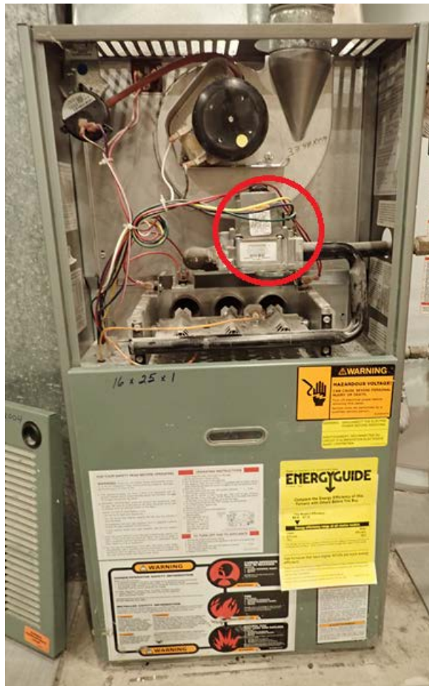
Figure 56. Example of the location of the gas solenoid valve in a residential furnace
