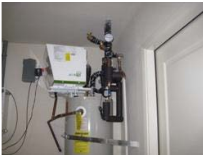
Figure 48. Omega FTB-4605 flow meter installed in a field test of a heat pump water heater
