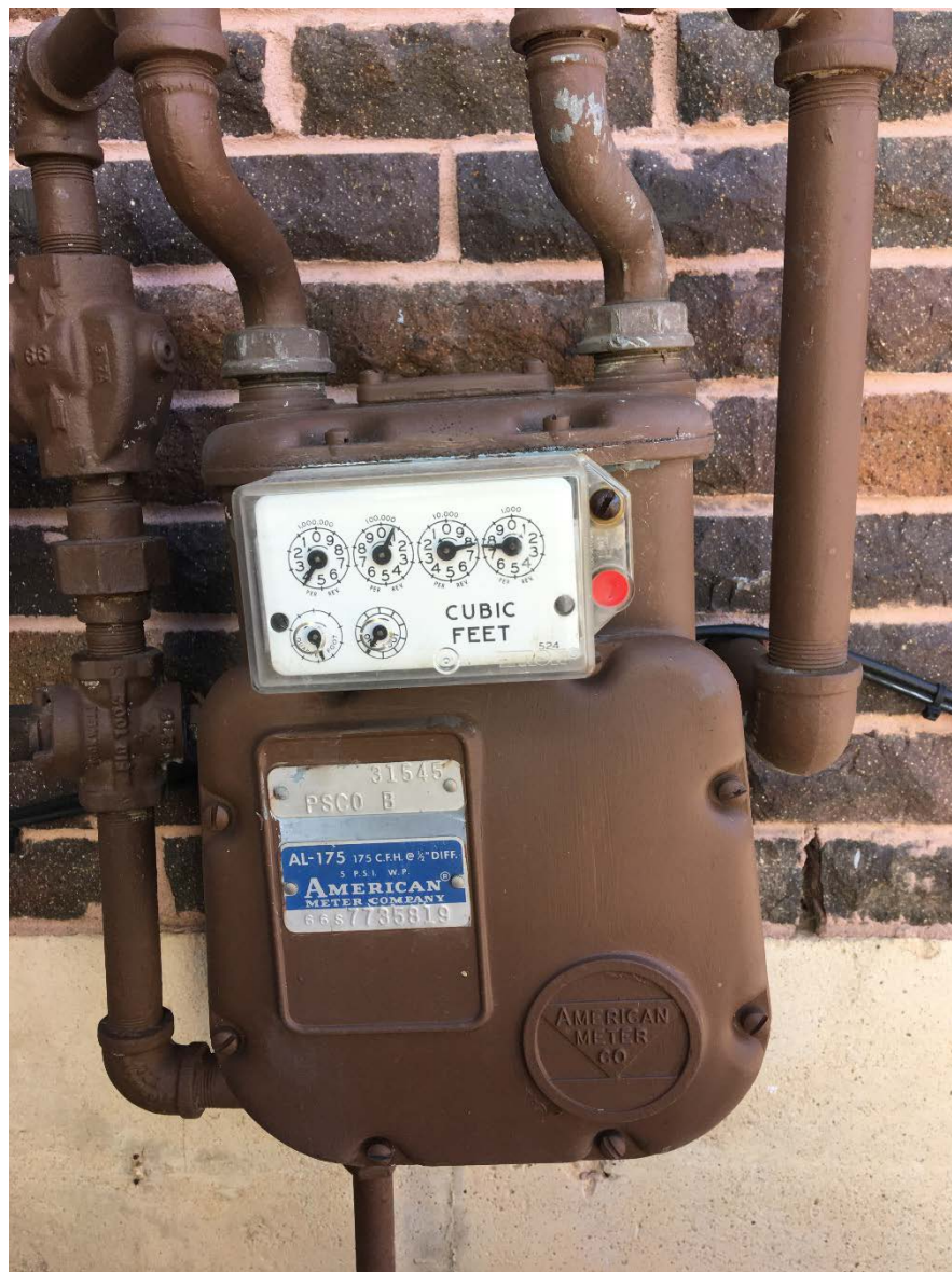
Figure 21. Typical residential utility gas meter
