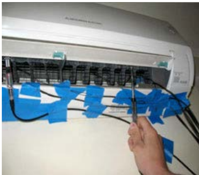
Figure 15. Hot wire anemometers used to measure airflow speed (installed on the left and handheld)
