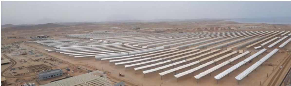
Figure 2. Ultimate Trough installed solar field in the KSA with a 170,000\text{-m}^2 total aperture area.
