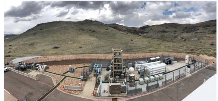
Hydrogen Infrastructure Testing and Research Facility (HITRF)
