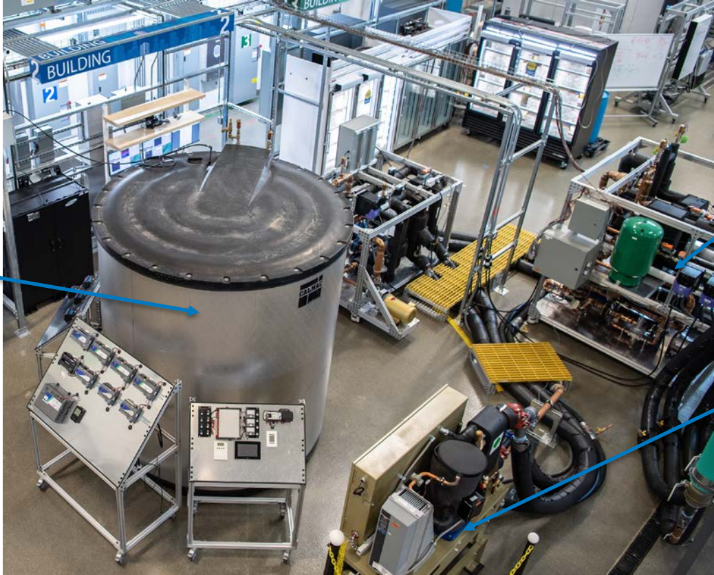
Ice tank, 162 tonh (570 kWh)
