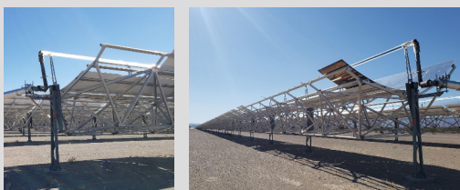
Parabolic trough rows at the Nevada Solar One (NSO) solar power plant with destroyed mirrors on the outer edge of the field. Photos by Ulrike Egerer, NREL
