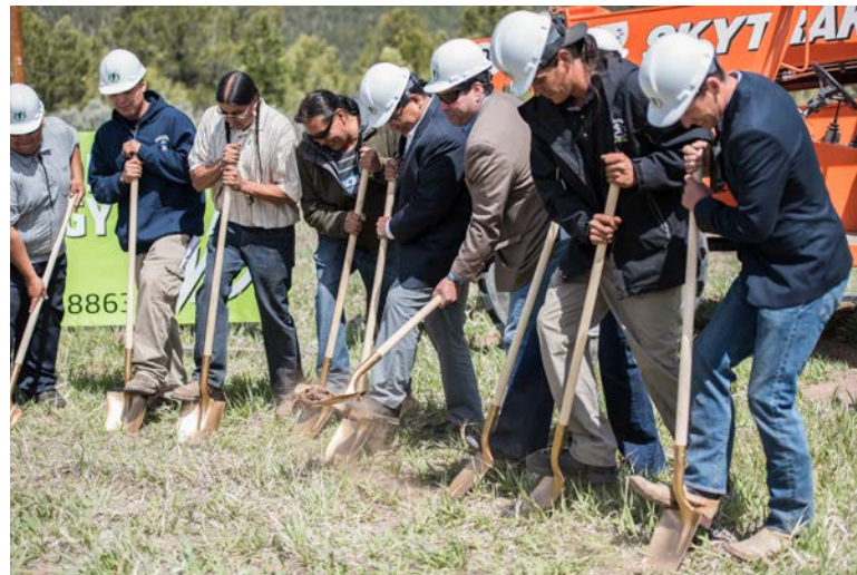
Breaking ground on a 1-MW array at Picuris Pueblo, NM. The cooperative, Kit Carson, works closely with the tribe.
