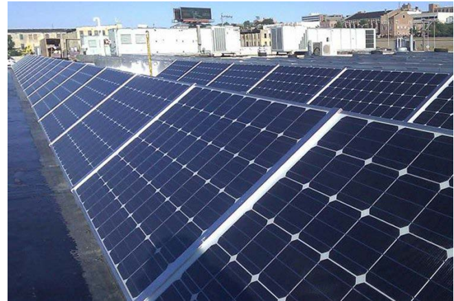
30-kW rooftop PV array that powers the Forest County Potawatomi Community administration building
