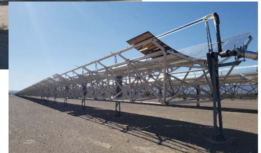
Parabolic trough rows at the Nevada Solar One (NSO) solar power plant with damaged mirrors on the outer edge of the field. Photos by Ulrike Egerer, NREL
