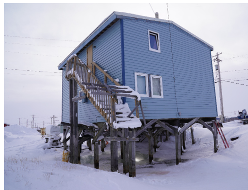
A building in Point Lay affected by permafrost thaw. Ground subsidence has left the stairs nearly seven feet off the ground, but because the piles have been driven so deep into the permafrost layer that the building is still standing and inhabited. Photo credit NREL.
