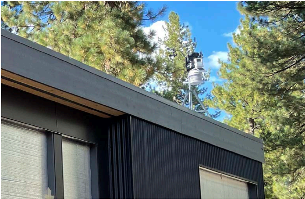
Figure 9. Weather station installed on top of the test home
