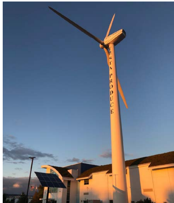
750 kW Aeronautica turbine installed at the Testa Produce warehouse in Chicago Photo from WES Engineering
