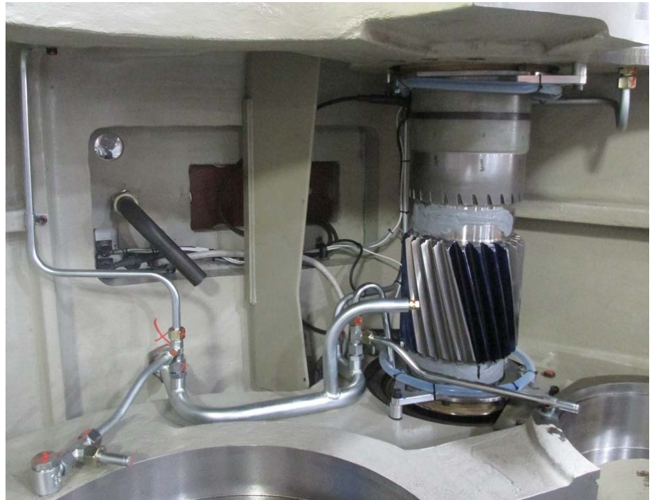
Photo by Shawn Doner, Flender Corporation, NREL 49750
