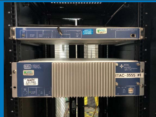
(b) Microgrid controller
