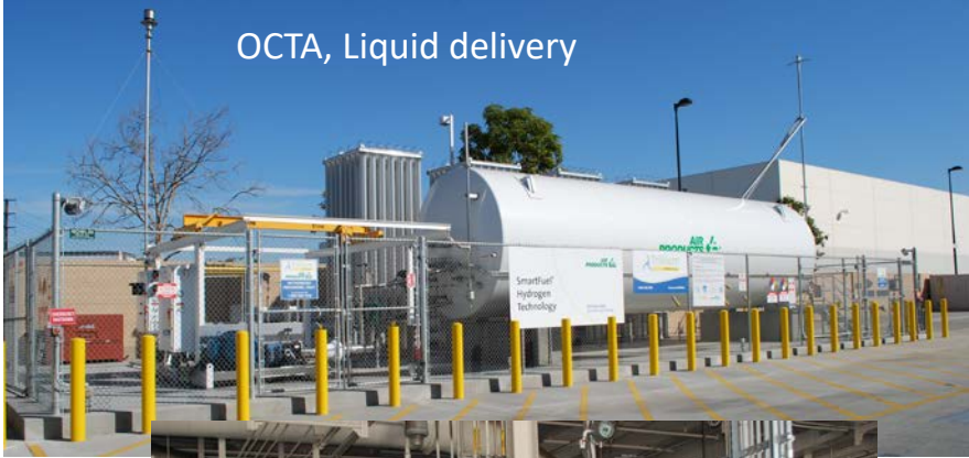
SunLine, on-site generation with electrolyzer
