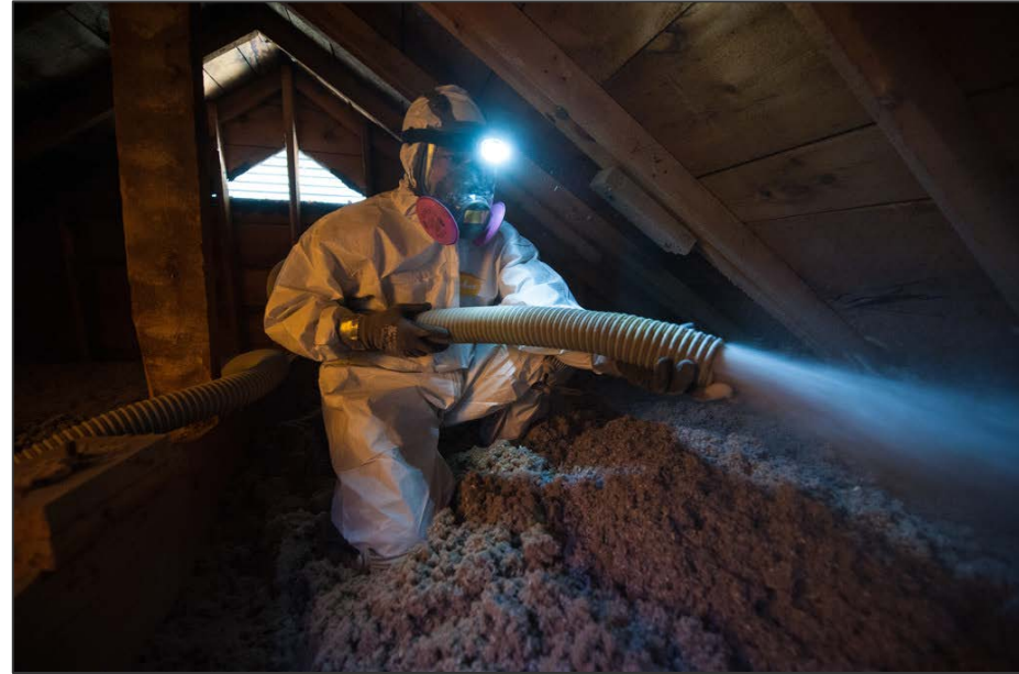
Photo from NREL image gallery 28767
