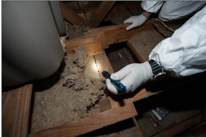
Photo from NREL image gallery 28560
