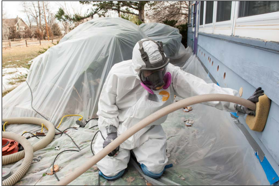
Photo from NREL image gallery 28786
