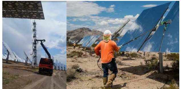
Figure 2. TRUCK WASHES LARGE HELIOSTAT AT CRESCENT DUNES (LEFT); WORKERS MANUALLY WASH HELIOSTATS AT IVANPAH (RIGHT). IMAGE SOURCE: [17]
