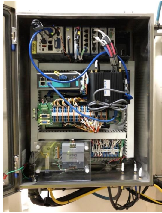
Fig. 6 Enclosure layout of a MODAQ field enclosure (Photo by Robert Raye, NREL)
