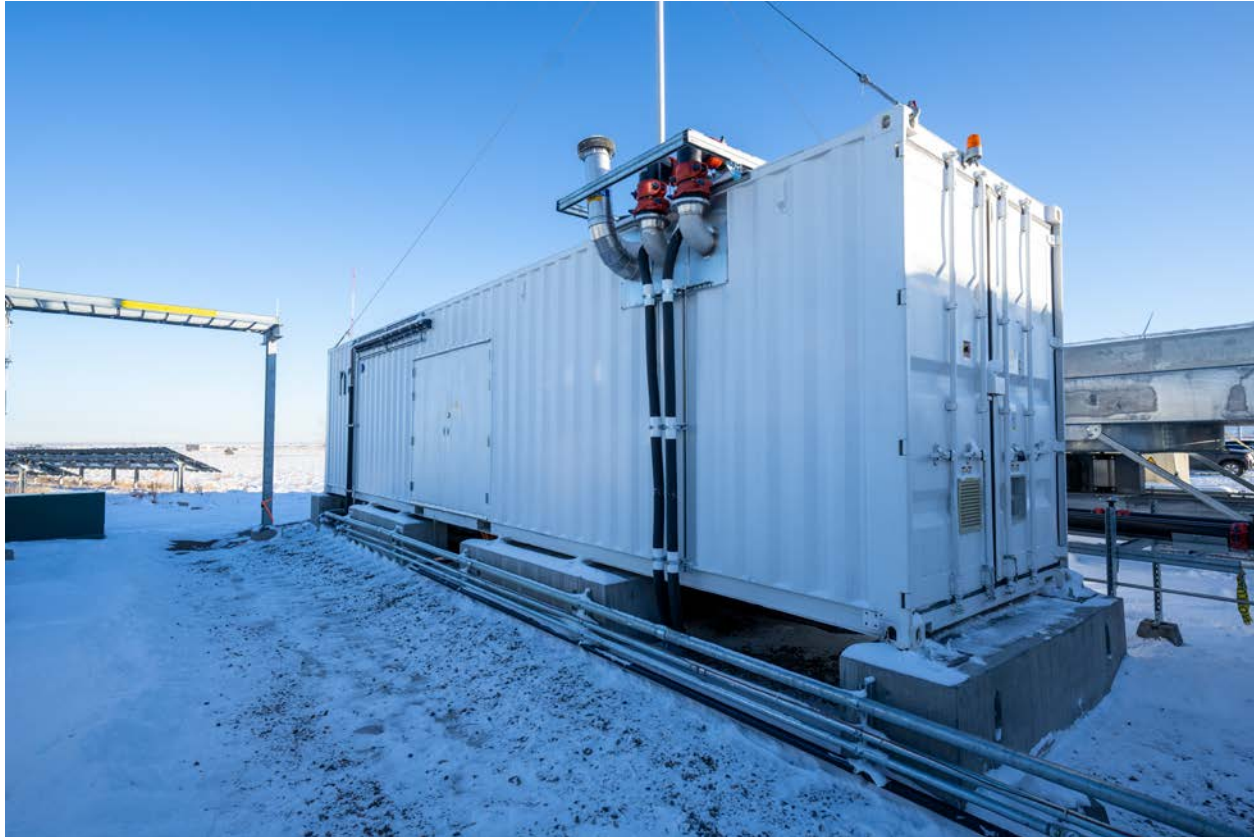
Photo by Werner Slocum, NREL - NREL image gallery image 74986
