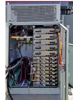
Vendor 3: 125 kW building block
