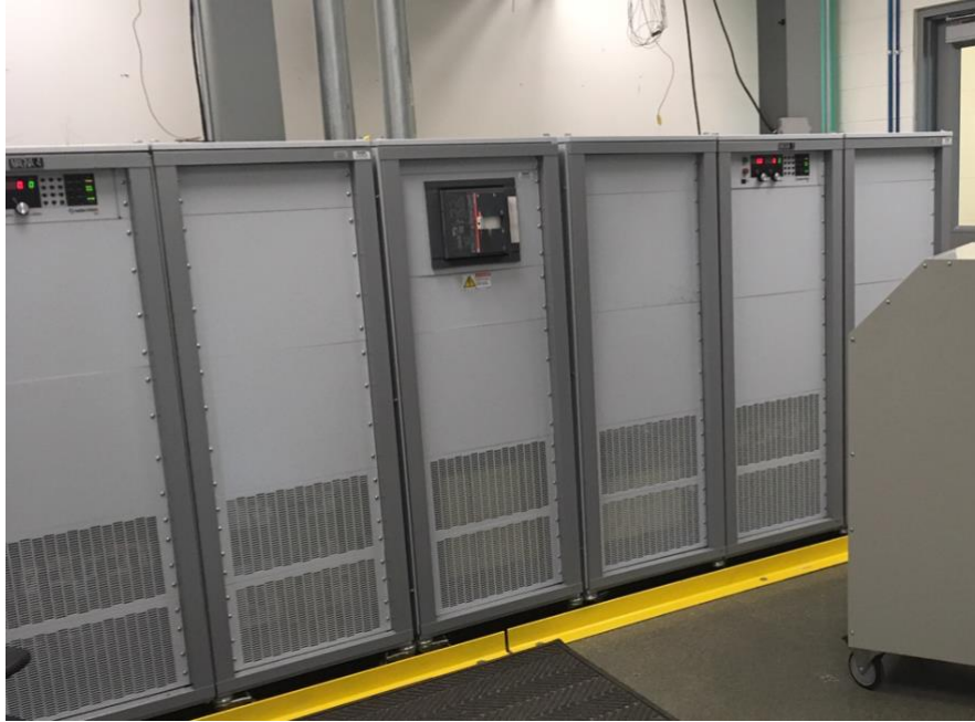
Figure 1. 500kW (out of 1MW) AC/DC power supplies at NREL power PEM electrolyzer system.
