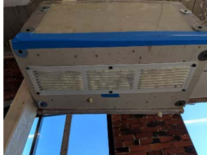
Figure 46. Foam bulging out of continuous soffit vents
