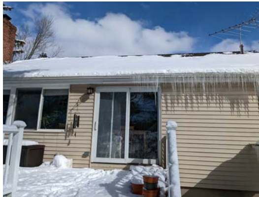
Figure 55. Ice formed on the uninjected (right) portion of the cathedral ceiling
