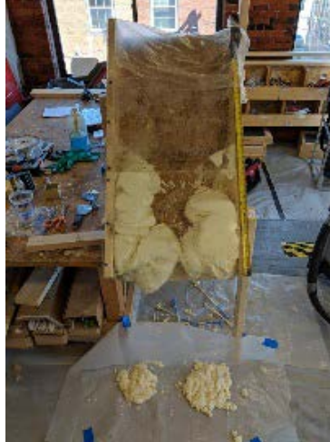
Figure 25. Blocking shot foam slumping into soffit space and onto floor
