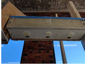
Figure 45. Foam bulging out of round soffit vents
