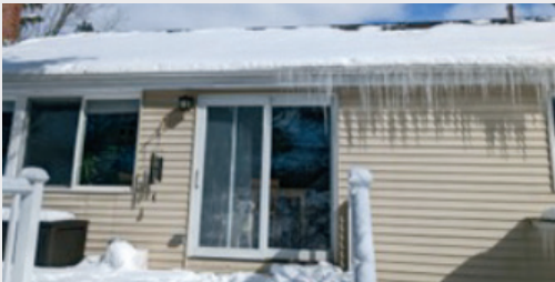
Figure ES-4. Ice formed on the uninjected (right) portion of the cathedral ceiling. No ice on the injected portion (left). Photo from the authors
