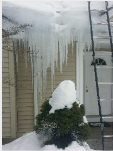
Figure ES-1. Ice dam in ERC Photo from the authors
