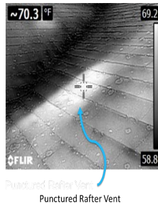
Figure 40. Hot spot on roof from punctured rafter vent
