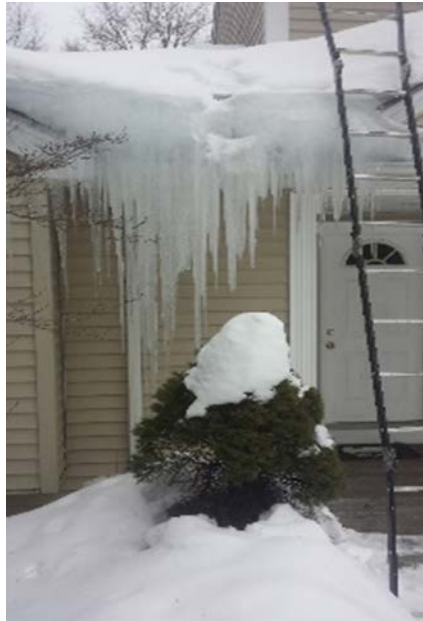
Figure 1. Ice dam in ERC
