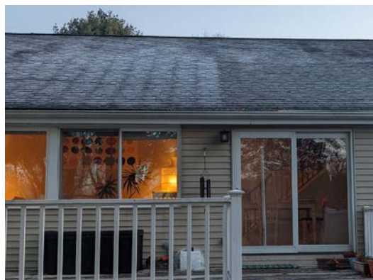
Figure 56. Frost formation on the injected (colder) side of the roof
