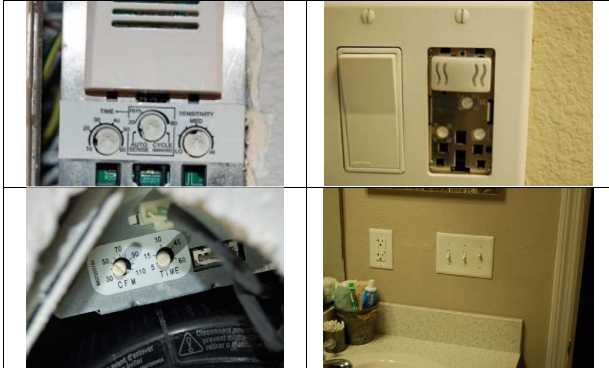
Figure 4. Examples of exhaust fan controls. Top – runtime and relative humidity controls located on switches. Bottom left – flow controls located on fan. Bottom right – wall switches that enable standard and boost operation.
