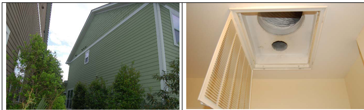
Figure 6. Left – CFIS outside air intakes high on wall are difficult to access for commissioning. Right – this return plenum ducting arrangement generates little flow through the 4-in. outside air duct.
