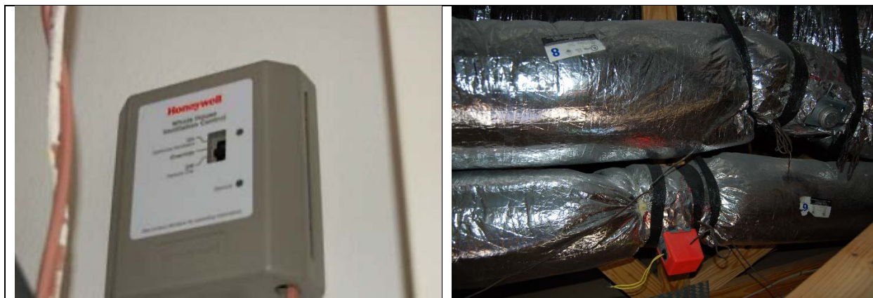
Figure 5. Left – common C-CFIS controller. Right – disconnected dampers prevent proper functioning
