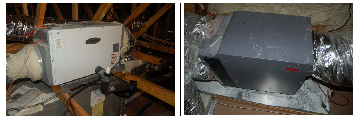
Figure 9. Left – the most commonly encountered dehumidifier processed outside air only. Right – one dehumidifier also processed air from the space. Both are ducted to central heating/cooling systems.
