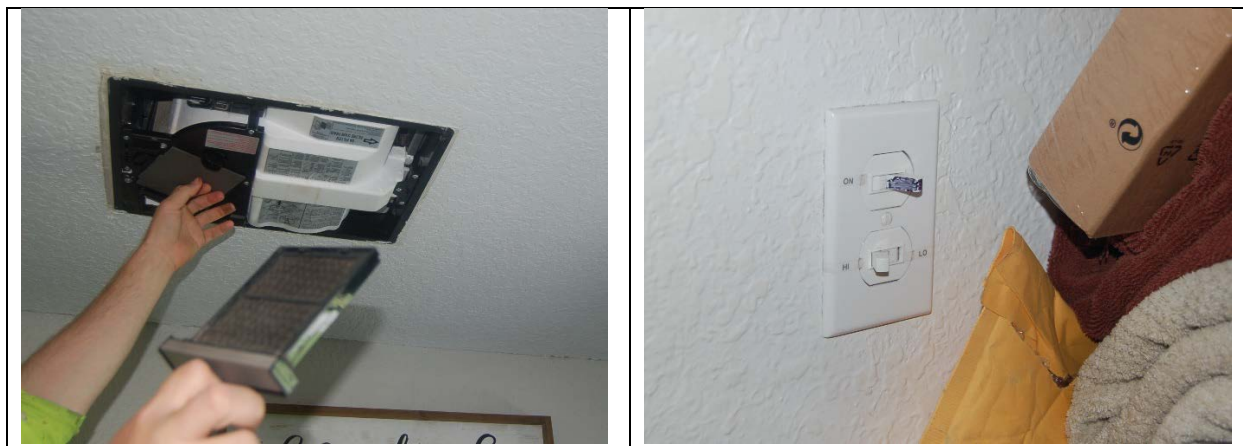
Figure 8. Ceiling-mounted ERV and associated wall switch controls
