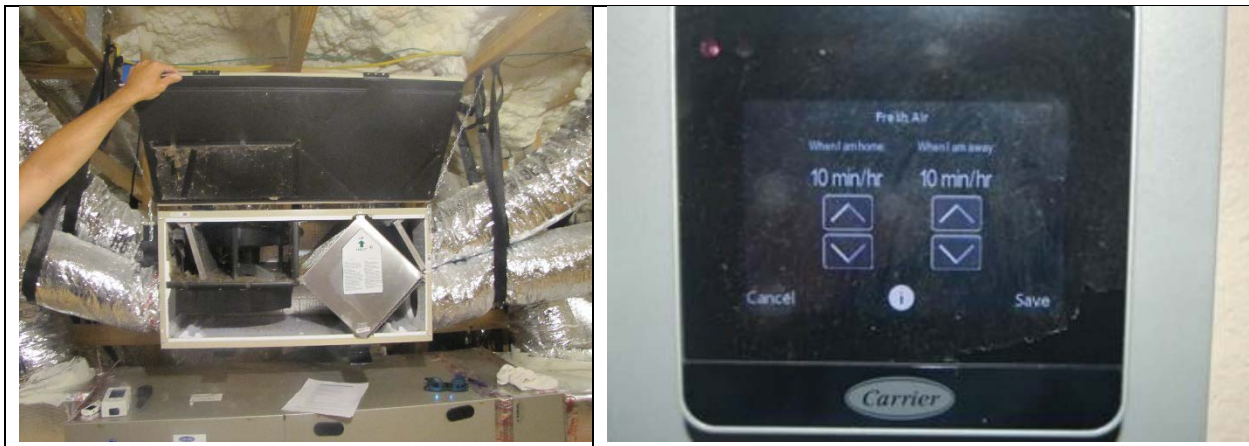
Figure 7. Left - attic-located ERV. Right - associated thermostat control. Dirty filter hindered operation.
