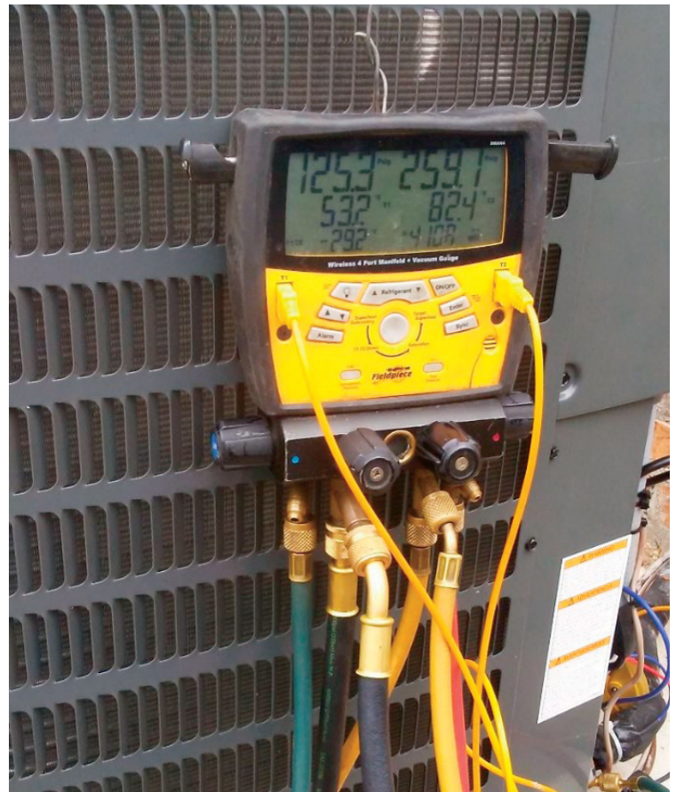
Example commissioning measurements. Photo from Home Innovation Research Labs
