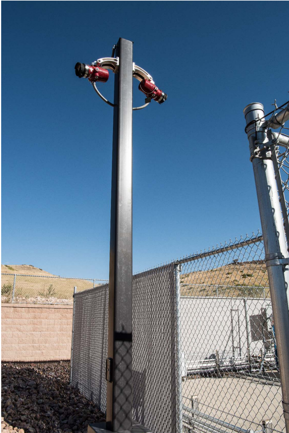
Figure 8. A flame detection system installed at NREL ESIF. Photo by Dennis Schroeder, NREL 40083.
