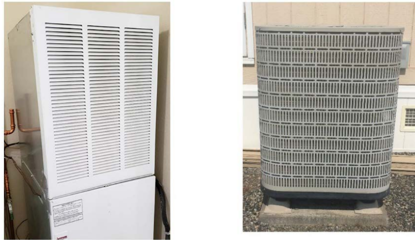
Figure 71. Heat pump indoor and outdoor units for the PNNL Lab Homes Photos from project team
