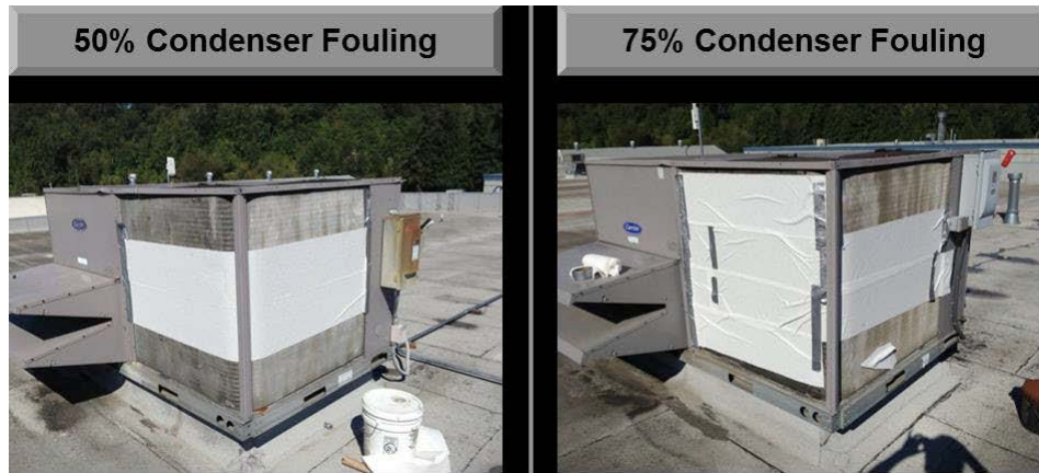
Figure 136. Condenser fouling implemented using paper
