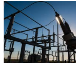
Source: NREL Flatiron Substation
