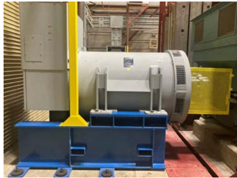
2MVA Synchronous Machine (driven by 2.5MW Dyno)
