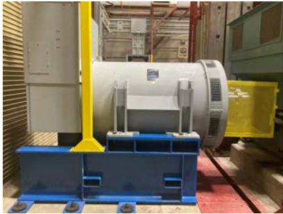
2MVA Synchronous Machine (Operating as a generator)
