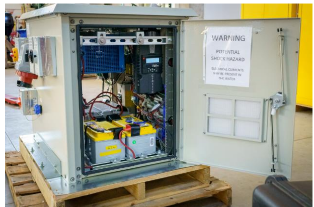
Fig. 3. A picture of the final power electronics enclosure that was deployed in North Carolina, USA, in 2022 (image credit: Andrew Simms, NREL)
