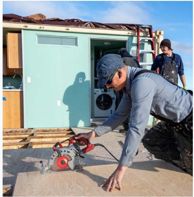
Local workers install floor decking after the placement of the kitchen/bath module. Photo by Vern Slocum, NREL
