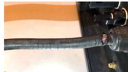
Cracking of tracker cable at the controller box.
