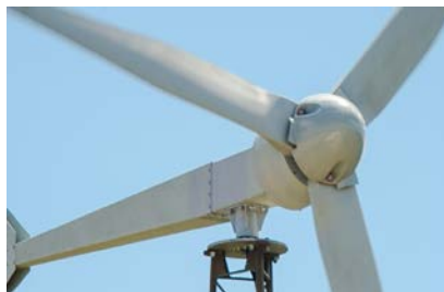
Bergey Excel 15-kW direct drive permanent magnet generator.
