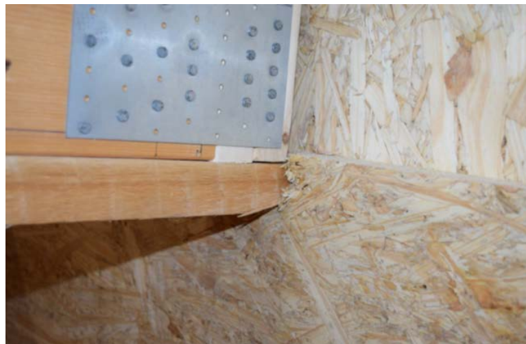
Figure A-18. Test 4 failure of joist/truss connection without splice joint movement or failure
