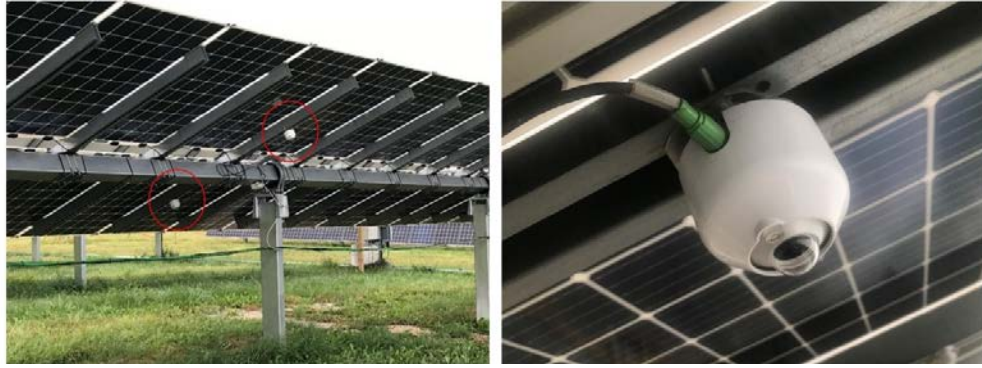
Figure 3-23. Example of multiple pyranometers (circled in red) used for RPOA monitoring of a south-facing, fixed-tilt BPV system (left). Close-up view of RPOA sensor mounting (right). Note that the array's length runs east-west and that the sensors are placed several meters away from the western or eastern array edges.
