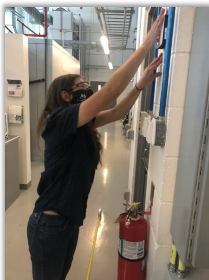
Figure 2. Installation of the sensor nodes in the ESIF's Systems Performance Laboratory on the NREL STM Campus. (Photo Credit: Otto Van Geet, NREL)
