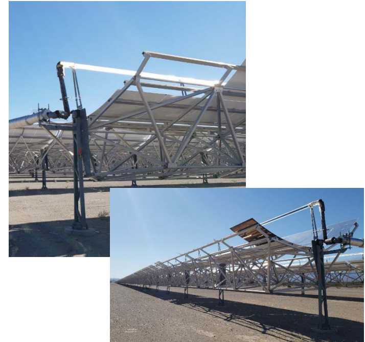
Parabolic trough rows at the Nevada Solar One (NSO) solar power plant with damaged mirrors on the outer edge of the field. Photos by Ulrike Egerer, NREL
