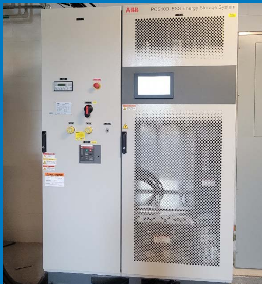
(a) Fuel cell inverter
