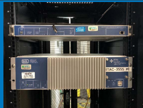
(b) Microgrid controller
