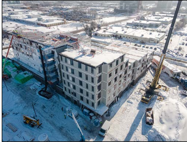
Figure 6. 200-unit commercial modular multifamily building in Minneapolis, Minnesota (Rise Modular project) for case study
