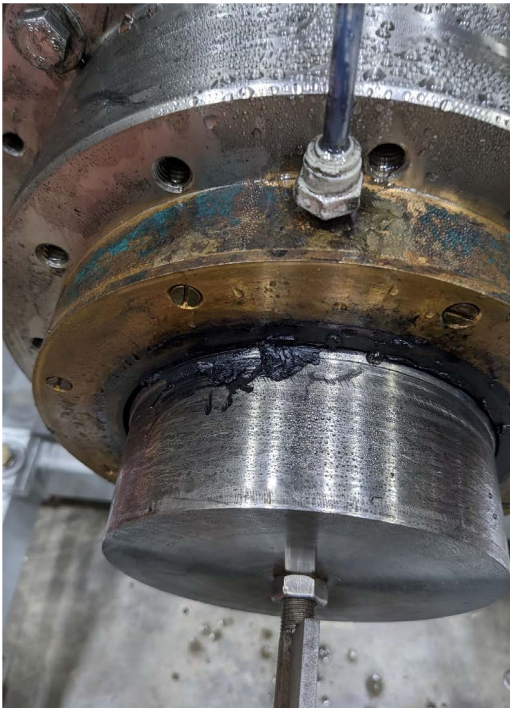
Figure A-2. Front of the MSS housing with water tank removed. A black paste can be seen extruding from the seal. The paste is a mixture of graphite and BF.
