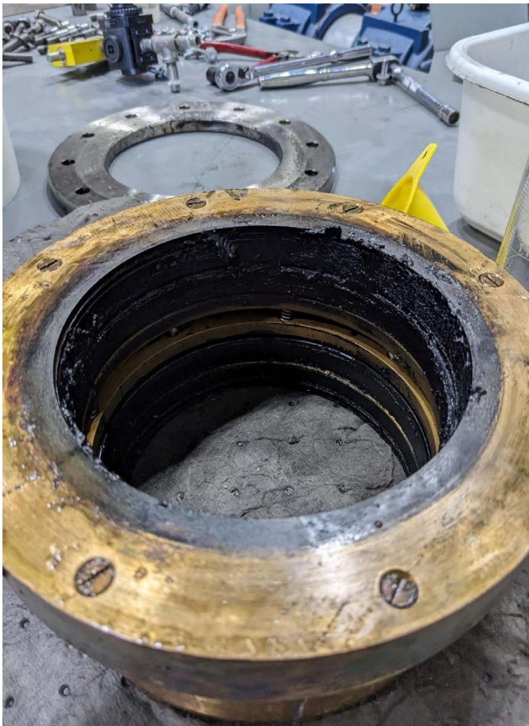
Figure A-4. MSS and housing removed from the shaft. The inside of the seal shows accumulation of graphite/BF paste. More accumulation can be seen at the front (top) of the seal than the back (bottom).
