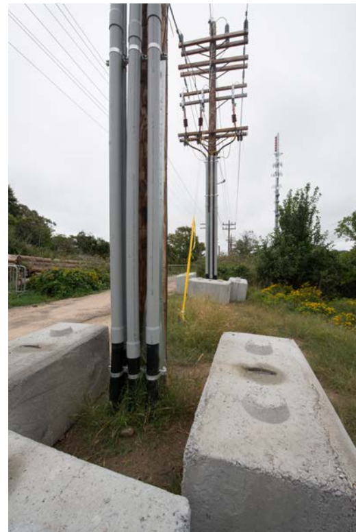
Upgraded grid infrastructure on Block Island. Photo by Dennis Schroeder, NREL, 40394
