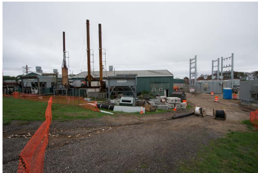
The old diesel power plant, left, was later replaced by the new switching station, right, for Block Island. Photo by Dennis Schroeder, NREL 40458
