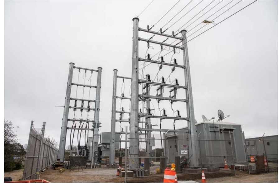
Transmission infrastructure on Block Island. Photo by Dennis Schroeder, NREL 40488
