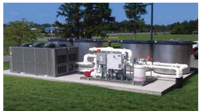
Figure 1. TES example: Ice tanks integrated with HVAC system. Image by Trane.
