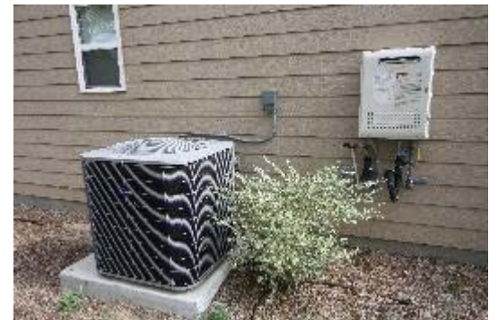
Ducted heat pump outside compressor. Image from Building America Solution Center
