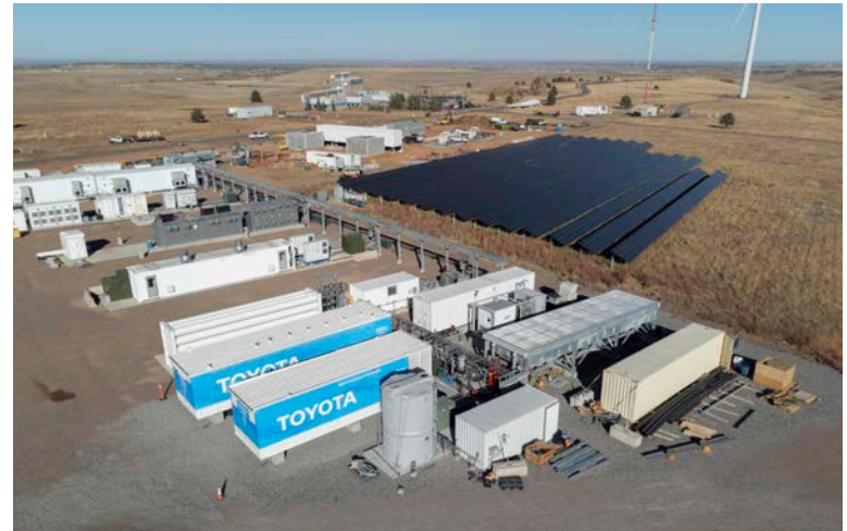
Hydrogen system at ARIES. Photo by NREL
