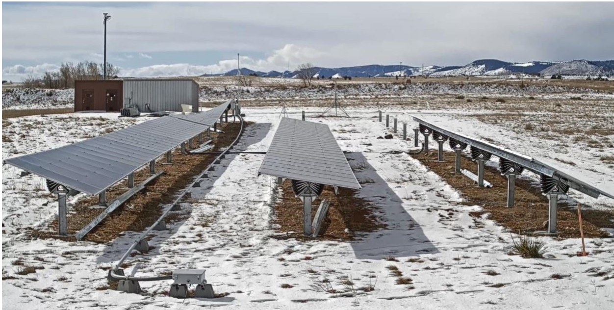
Figure 11. Screenshot of video under high wind. Note the early A90 generation of technology without dampers on top left showing deformed shaped due to dynamics under high wind (compare with Figure 5)
