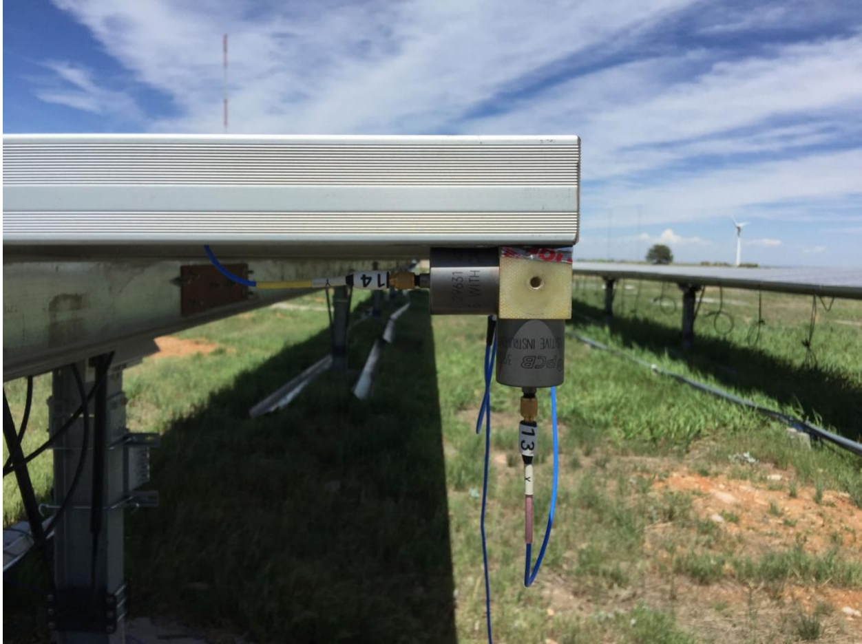
Figure 14. Close up of one of the biaxial accelerometer installations
