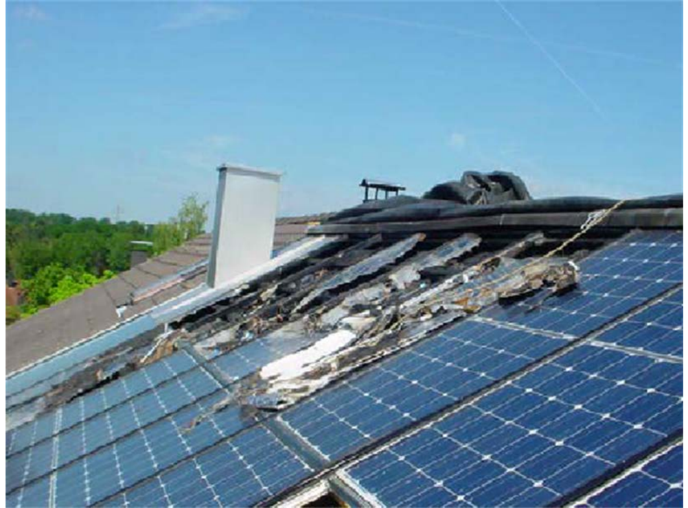
Roof fire caused by ground fault
