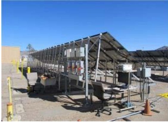
Test set-up used at DETL of SNL
