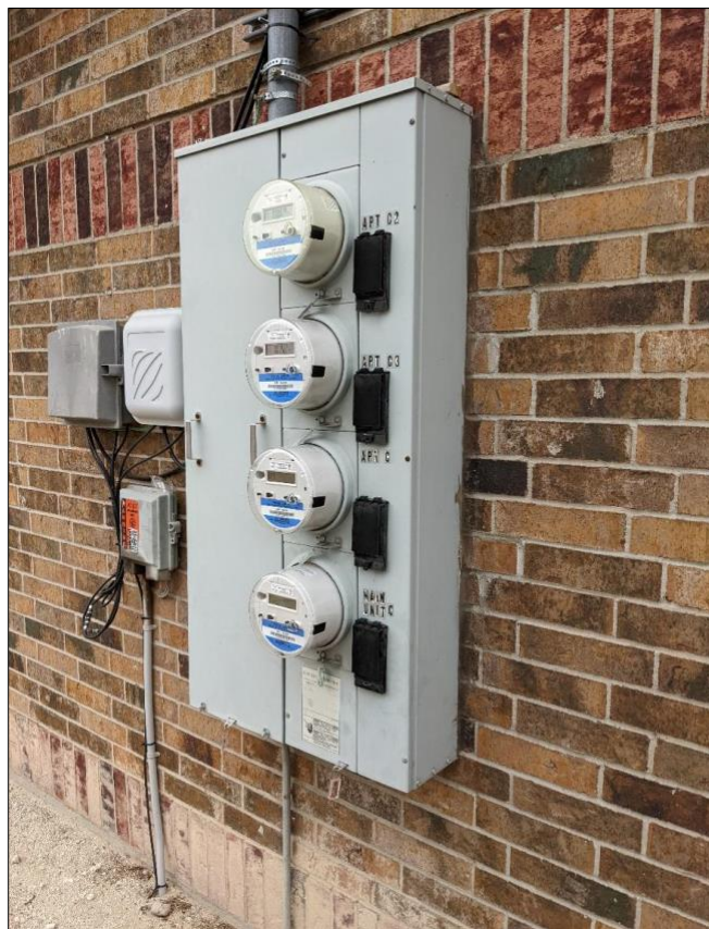
Figure 6. Building C meter bank—note additional meter for common area loads. Left side of panel is locked by the utility.
