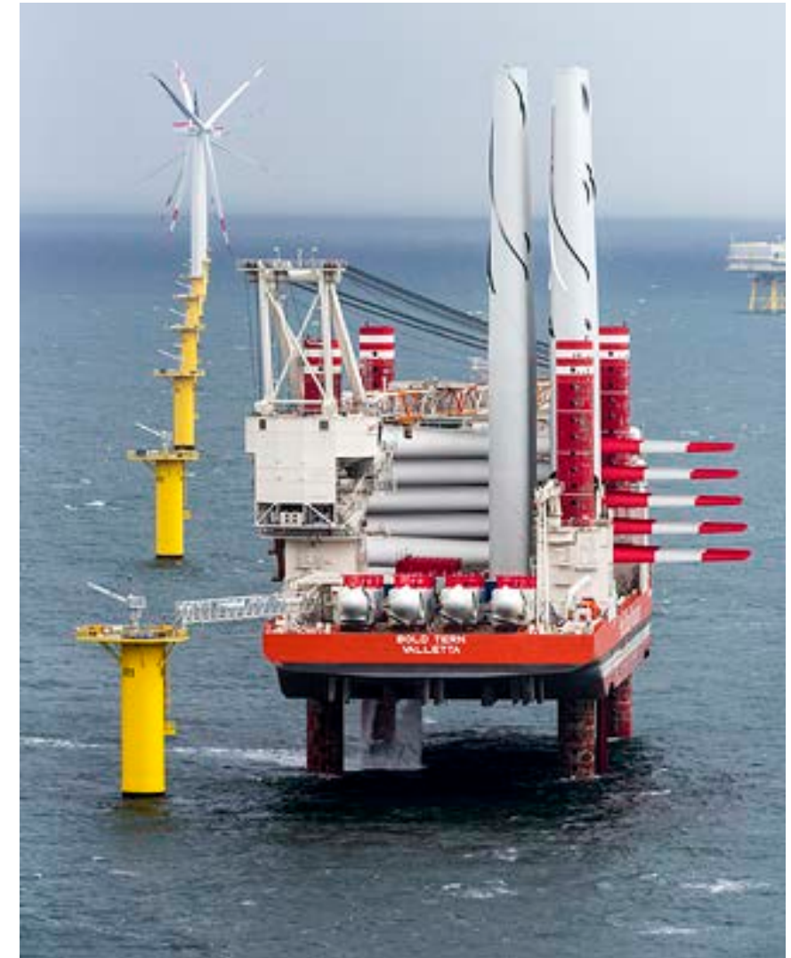
Figure. A jack-up barge at the Borkum Riffgat Offshore Wind Farm in the North Sea, Germany
