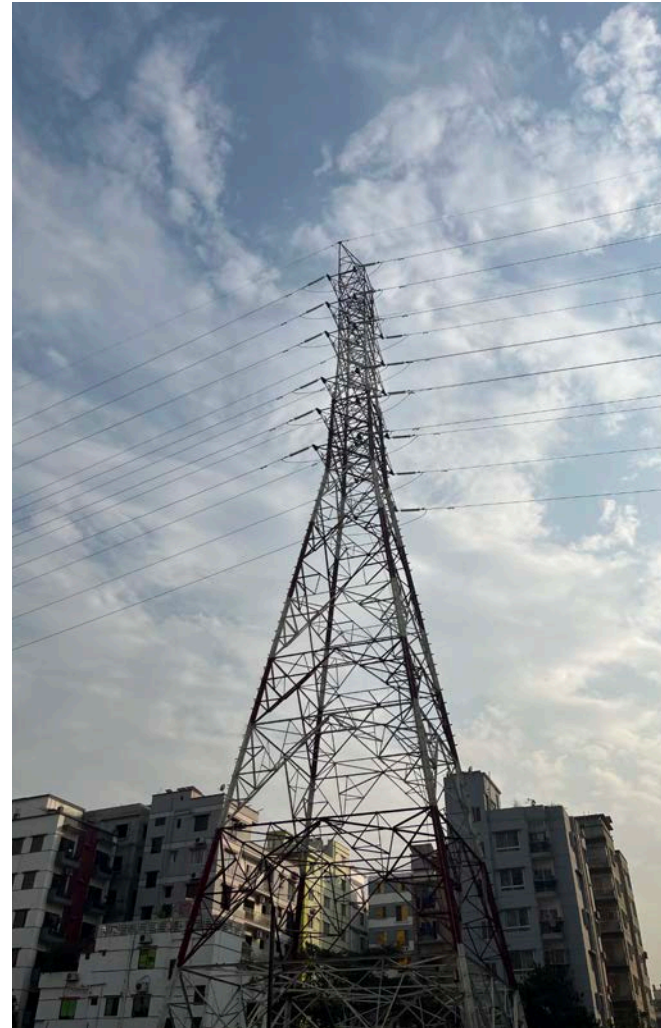
Figure. High voltage AC transmission lines near the office of the Power Grid Corporation of Bangladesh
