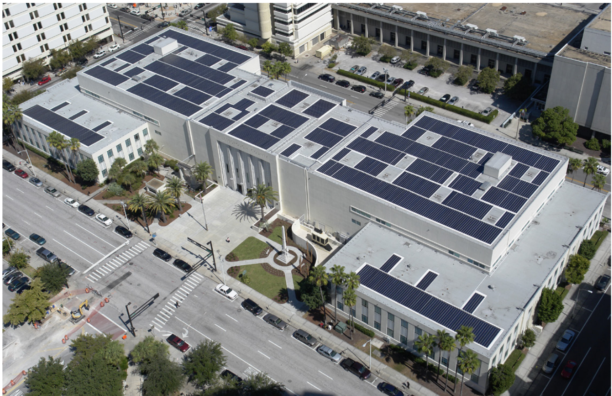
196-kW rooftop photovoltaic system at the Hillsborough County Courthouse (Credit: Hillsborough County)
