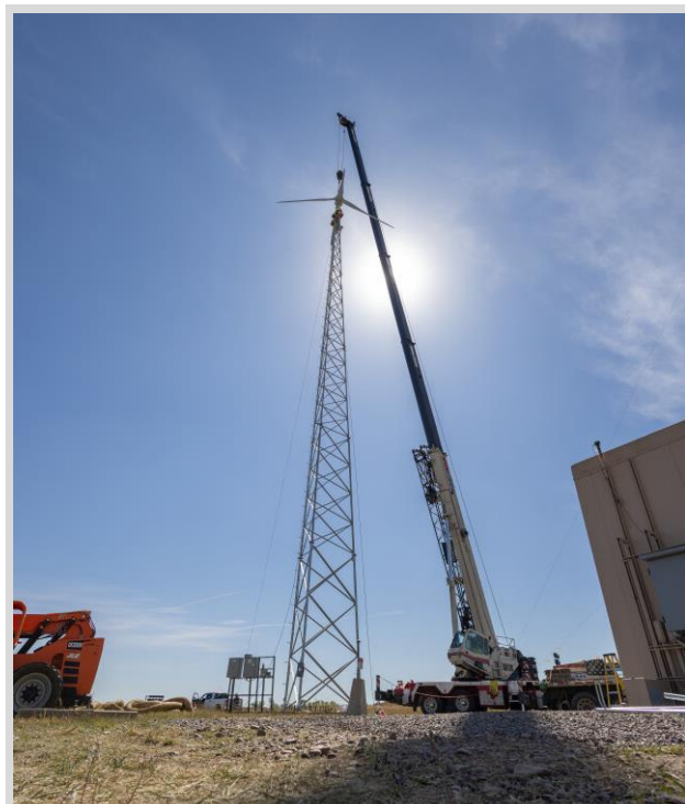
Crews install a Bergey Windpower Excel 15 wind turbine at NREL's Flatirons Campus distributed wind energy site. Photo by Joe DelNero, NREL
