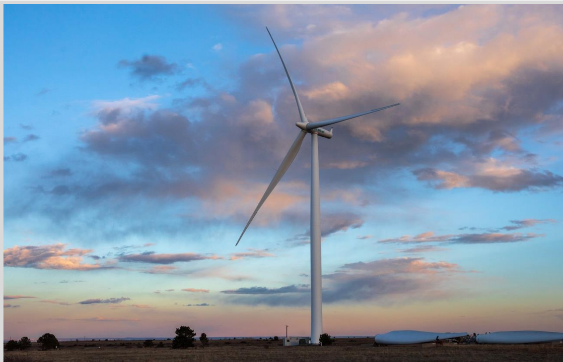
NREL is negotiating with Siemens Gamesa to take ownership of the 2.3-MW wind turbine at NREL's Flatirons Campus shown here. Photo by Werner Slocum, NREL
