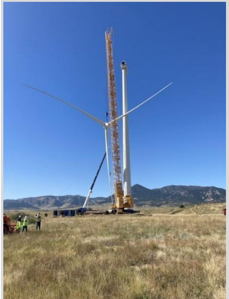
After 12 years of controls, drivetrain, and grid integration research, the Siemens Gamesa 2-MW G97 wind turbine was removed from NREL's Flatirons Campus. Photo by Jeroen van Dam, NREL
