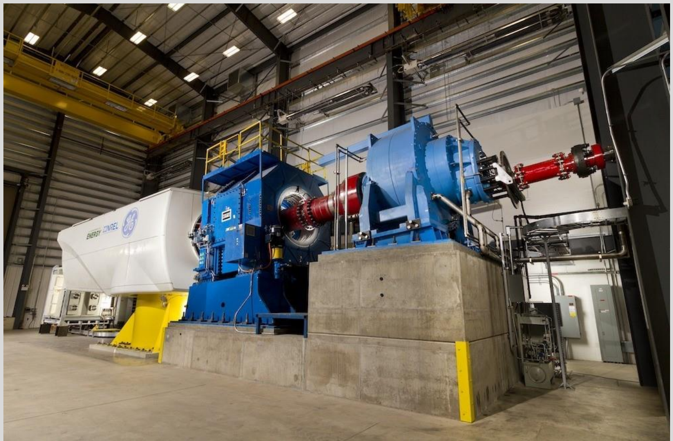
Researchers subjected GE's 2.5-MW wind turbine drivetrain, shown here attached to NREL's 5-MW dynamometer, to grid faults to test its stability in grid-forming mode. Composite photo by Pat Corkery, Mark McDade, and Dennis Schroeder, NREL
