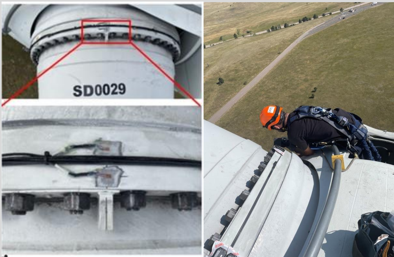
Strain gauges installed on a pitch bearing of the DOE 1.5-MW wind turbine on NREL's Flatirons Campus will yield insights into pitch bearing reliability. Photos from Jesse Graeter, Onyx Insight 85947 (left) and 85940
